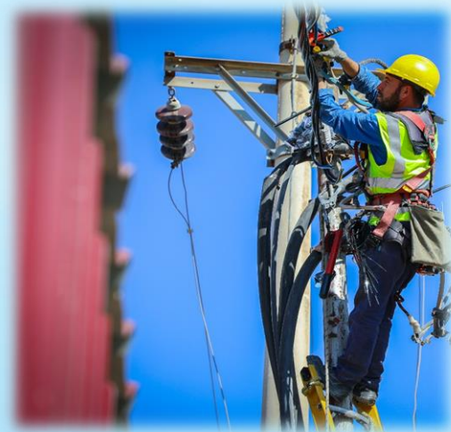
Added Low Voltage Network lengths 174.7 KM
